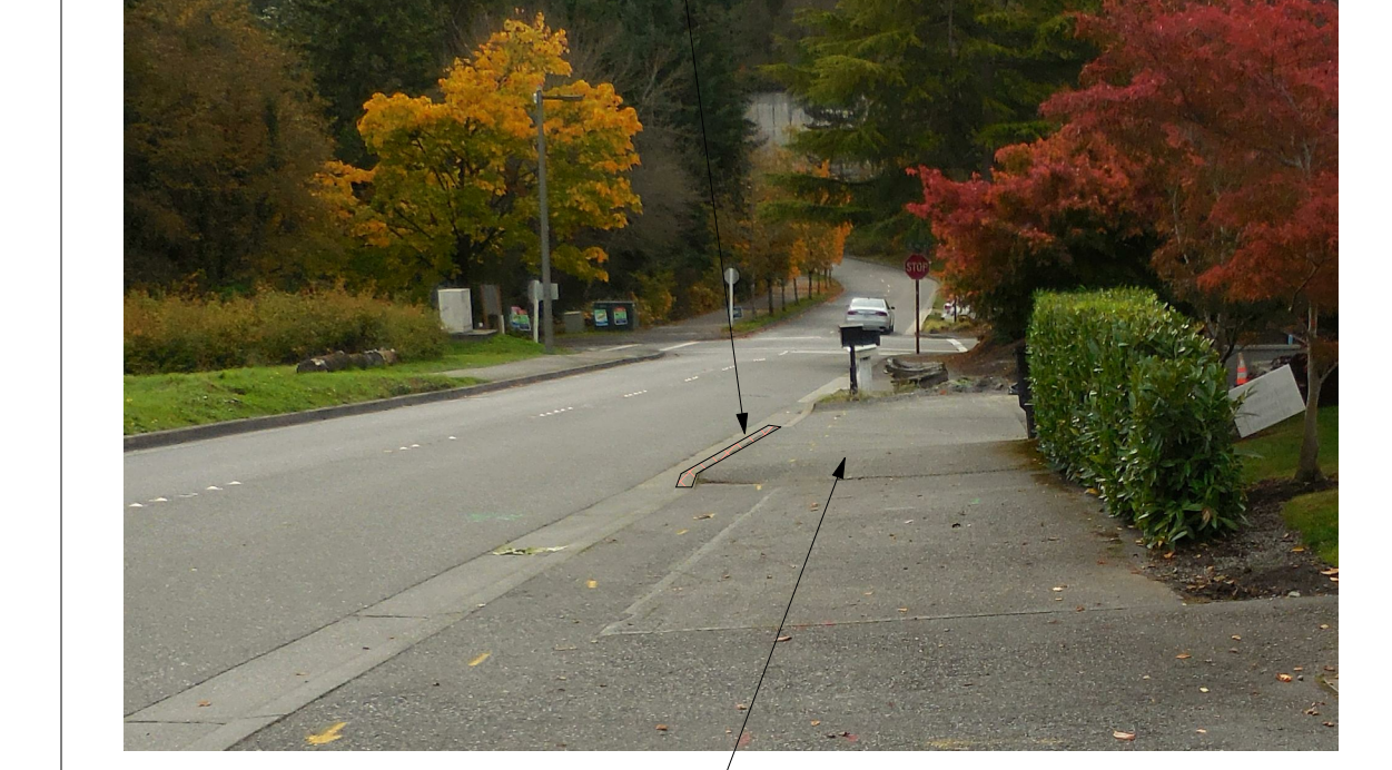
REMOVE EXISTING ELEVATED SIDEWALK AND REGRADE TO MATCH ADJACENT GRADING TO MEET NEW BACK OF CURB HEIGHT.
